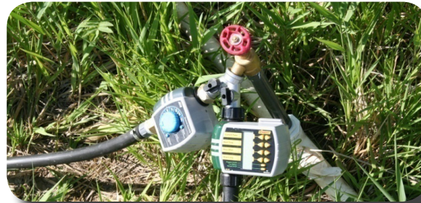
Solar Powered Irrigation System
